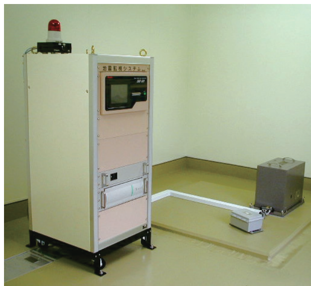
図1 新幹線早期警報用地震計の設置状況 Fig.1 Seismograph of earthquake early warning system for railway
